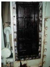
Oily inside of oil water separator
