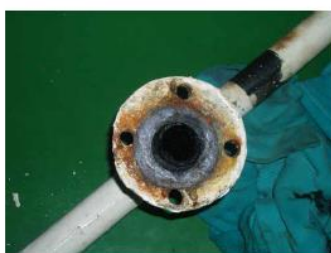
Oily inside of discharge pipe
