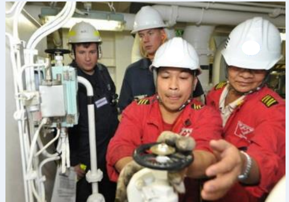
[Photo: ‘US Coast Guard’ Two engineers as they test the oily water separator in the vessel’s engine space during a port state control exam]
